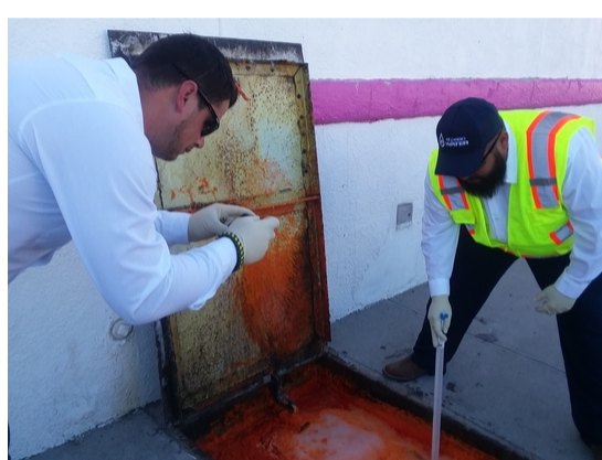
Pretreatment Inspector Supervisor Kyle Eckert documents a local bakery's grease trap, with the assistance of Pretreatment Inspector Luis Velasquez.
